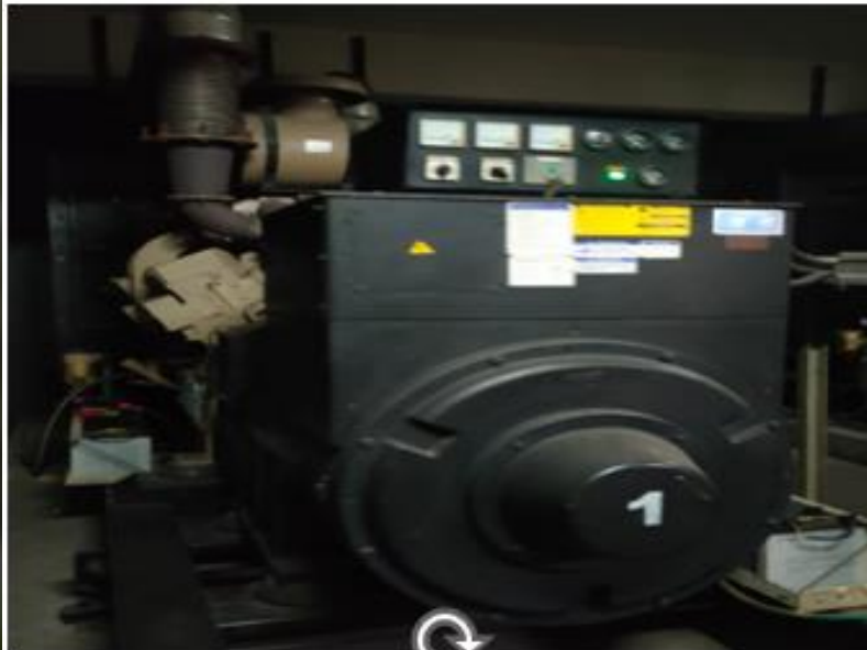
Genset Perlu Service
