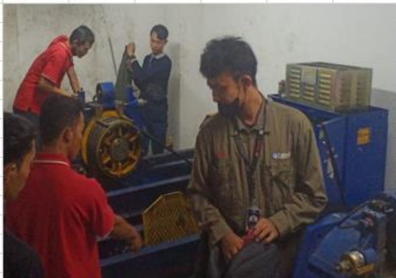
Overhault Lift P2
