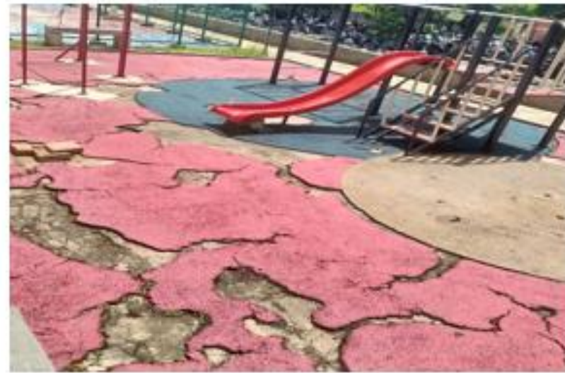
LANTAI PLAY GROUD RUSAK
