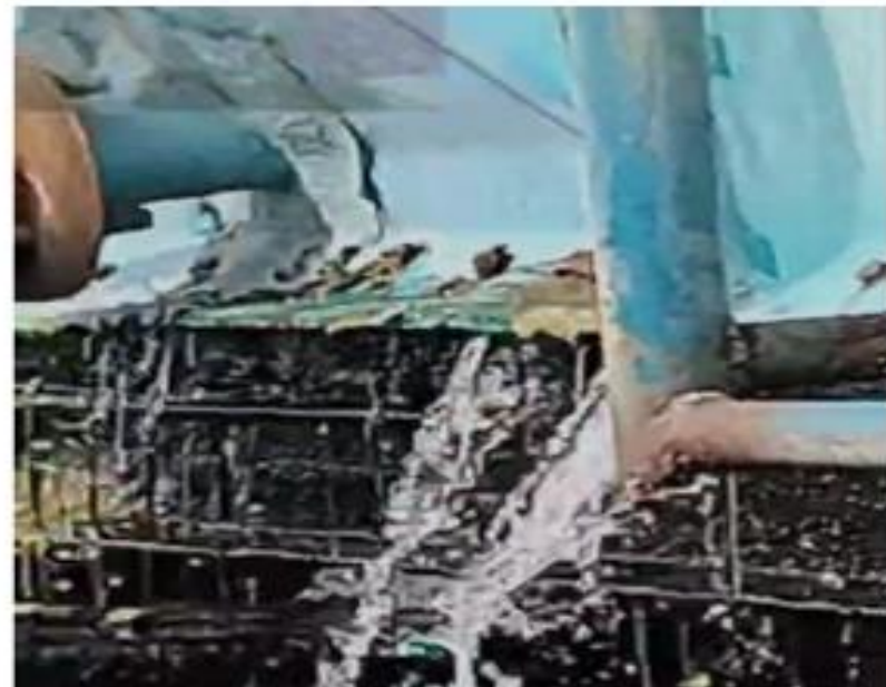
Roof Tank Bocor
