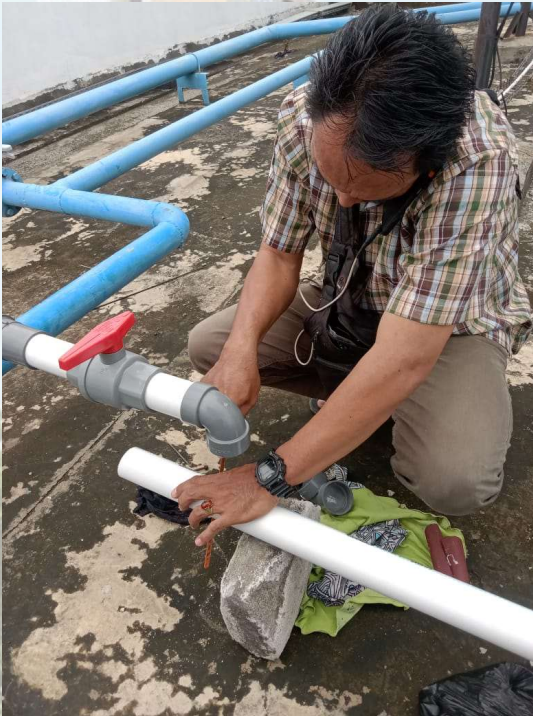
● PERMASALAHAN : Roof Tank Tower Ruby
